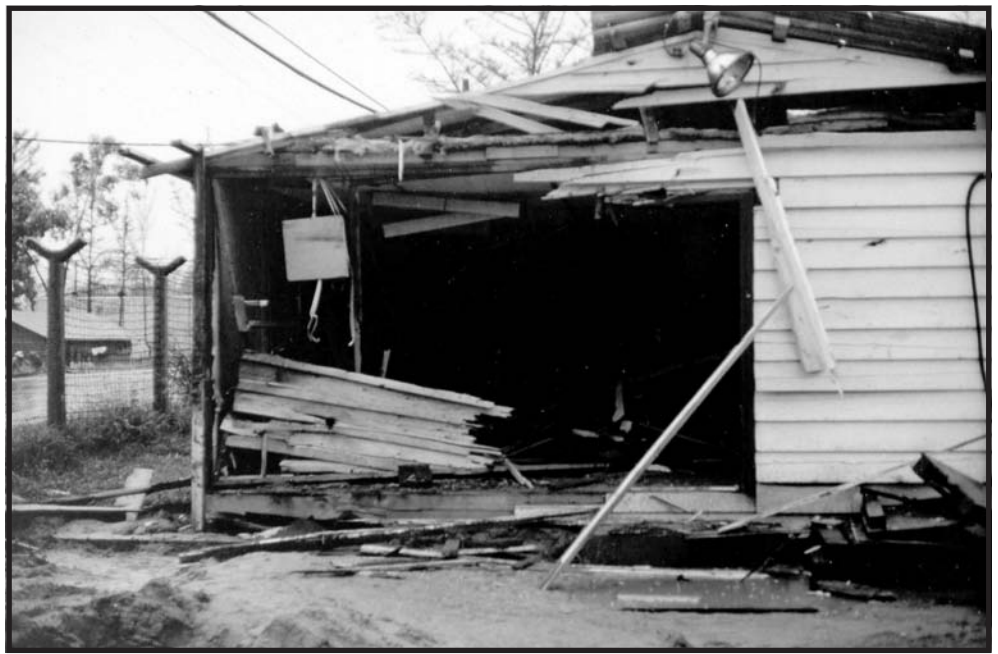
Combined Detachment DaNang Intelligence office, mission/SI briefing/debriefing area and NSG equipment shop damaged by a near direct hit of a rocket circa 1968.
